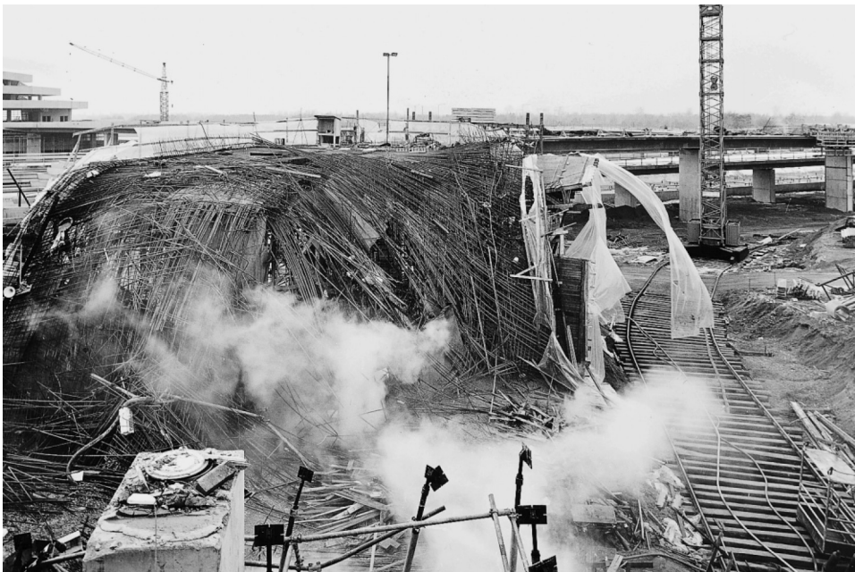
Fig. 11.1 Collapse of supporting scaffolding for a bridge ramp at Cologne-Wahn airport. 1995, Case 11.45
