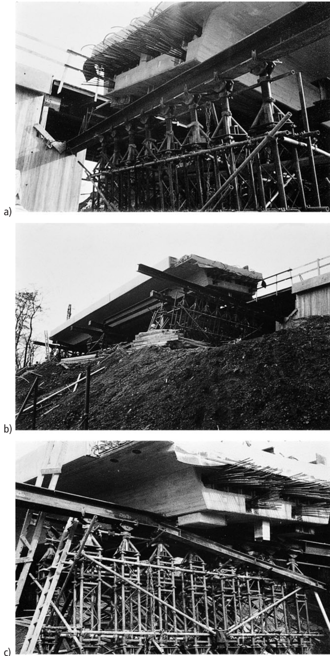
Fig. 11.6 Scene of partial collapse of a railway bridge between Solingen and Ohligs during sideways jacking, 1977, Case 11.29
